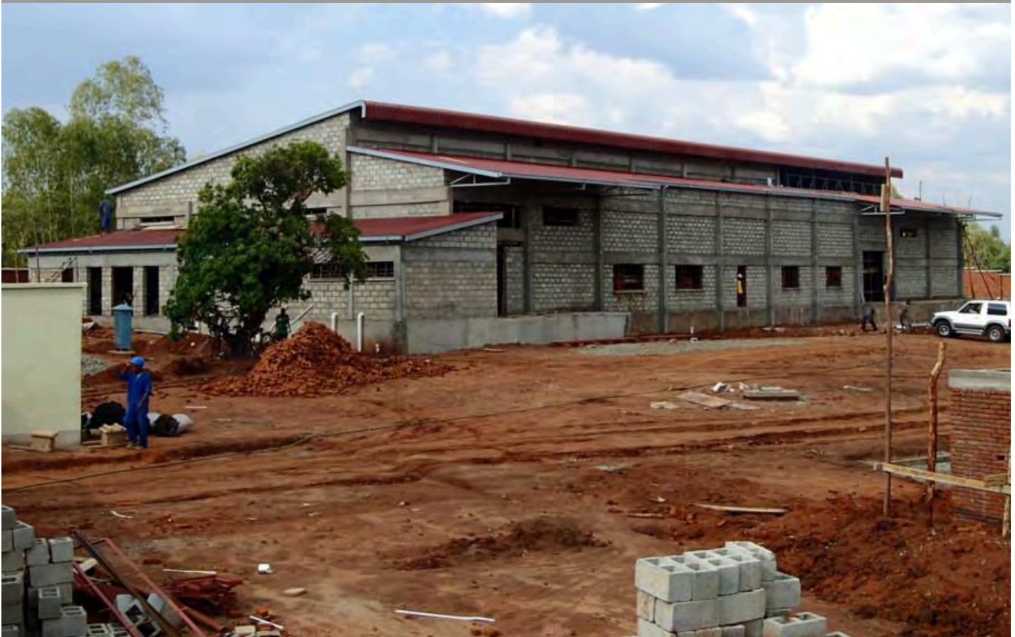
Above: An exciting glimpse of the new factory building in Blantyre, Malawi. The team hopes to begin moving production machinery and personnel to the new site in March 2014.
